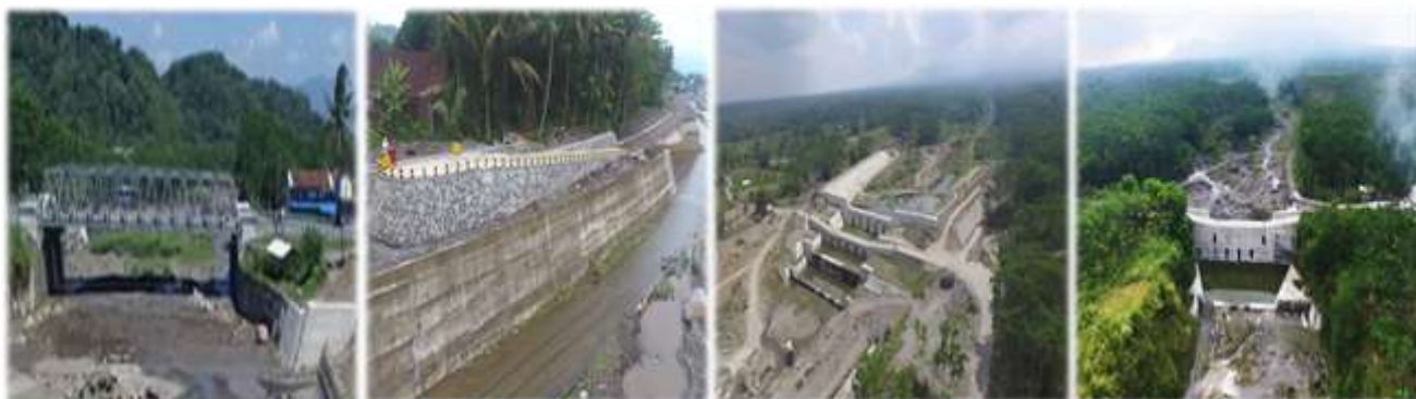
Gambar 2.6. Dokumentasi Kunjungan ke Lokasi Proyek Urgent Disaster Reduction for Mount Merapi and Lower Progo River Area
